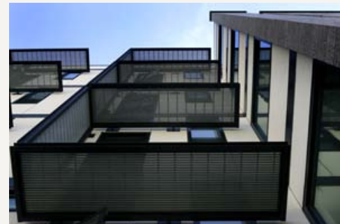
Sunscreens make the windows of the student housing facility even more energy efficient. Download photo
